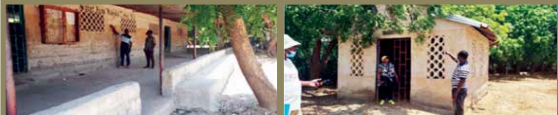
Plate 3: The height of flood waters that befell St. Kelvin's School, Lodwar Town. The waters were observed at 3m above ground level.
